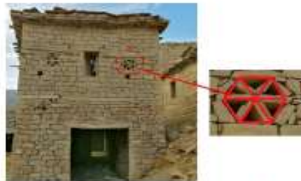
Figure 8. Habitat apertures of the vernacular Auresian architecture of the Oued Abdi valley
