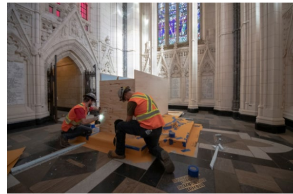
Figure 5.15. Workers install plywood to protect the First World War altar in the Memorial Chamber (Source: Public Services and Procurement Canada, 2021)
