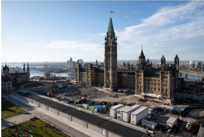
Figure 5.7. The construction site outside the Centre Block, as seen from the East Block, in November 2020 (Source: Public Services and Procurement Canada, 2021)
