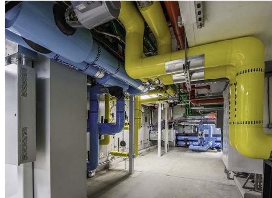
Figure 5.9. Basement Mechanical Room after restoration. (Source: Courtesy of Westlake Reed Leskosky,2019)
