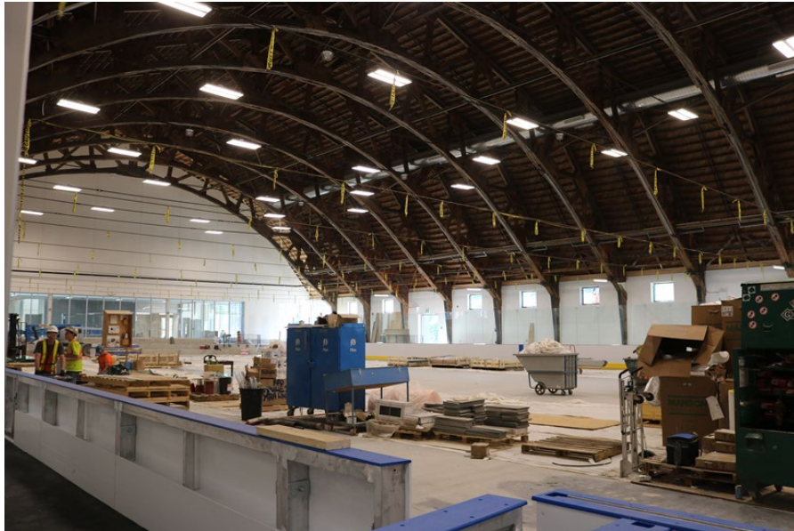
Figure 5.11. The arena under renovation with retaining the distinctive wooden roof truss system (Source: https://www.oakville.ca/townhall/oakville-arena-redevelopment.html )
