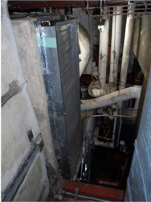
Figure 5.8. Pre-Renovation Condition of the Mechanical Room. (Source: Courtesy of Westlake Reed Leskosky,2019)
