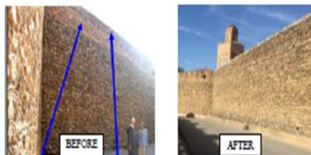
Fig. 8: The rampart before and after restoration, Source: The National Office for the Management and Exploration of Protected Cultural Property (OGEBP), Tlemcen
