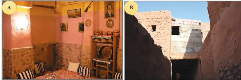
Figure 9. Use of standardized materials not compatible with the material, earth: A) the barrier that prevents the earth breathing; B) overloads that weaken the structure [22].
