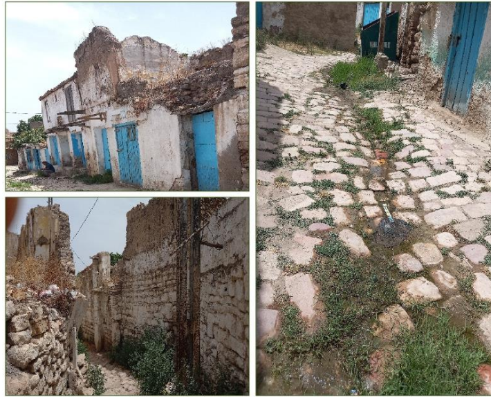
Figure (6,7,8). Architectural and urban degradation. Source: Authors, July 2021.
