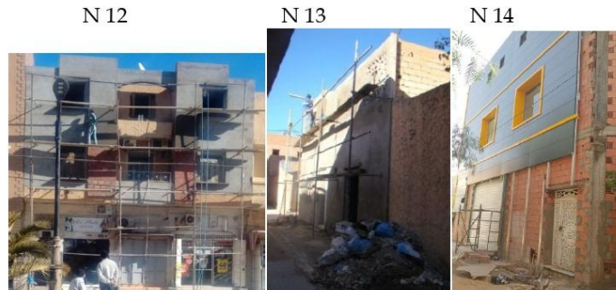
Photos 12-16: Individual residential samples showing construction interventions at the facade level in Qanani neighbourhood
