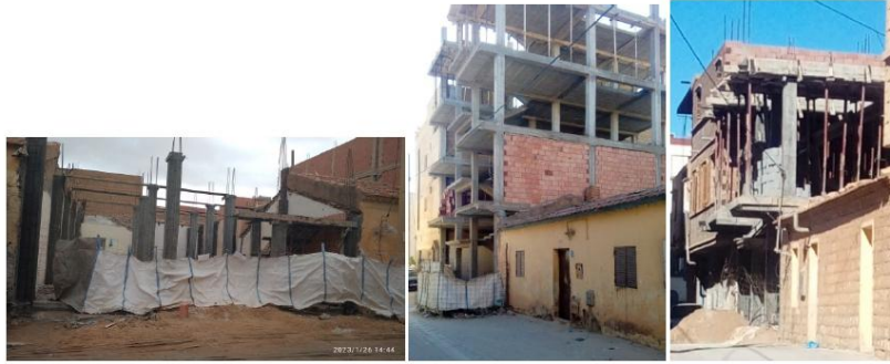
Photos 3-5: Demolition of traditional housing and reconstruction Source: Researchers, Residential samples, Qanani neighborhood. 2023.2022
